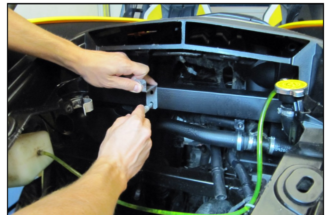
18. Using one of the Rear Brackets (#11) and a spring loaded punch, mark the cross member at both 3" marks. The Brackets are slotted for minor vertical adjustment.
